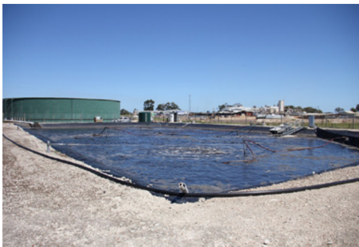
Figure 1B. The aerated pond wastewater treatment system at DBC during the ammonia oxidation phase
