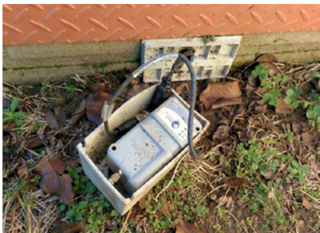
Figure 4. Vandalism at Schools
