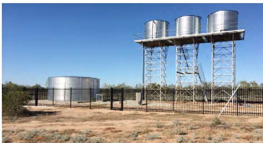
Recent infrastructure upgrades in one Aboriginal community. The Aboriginal Communities Water and Sewerage Program ensures ongoing operations, maintenance and monitoring of infrastructure.
