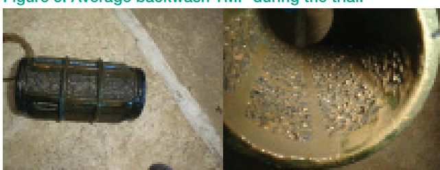
Figure 6. Screen filter before cleaning.
