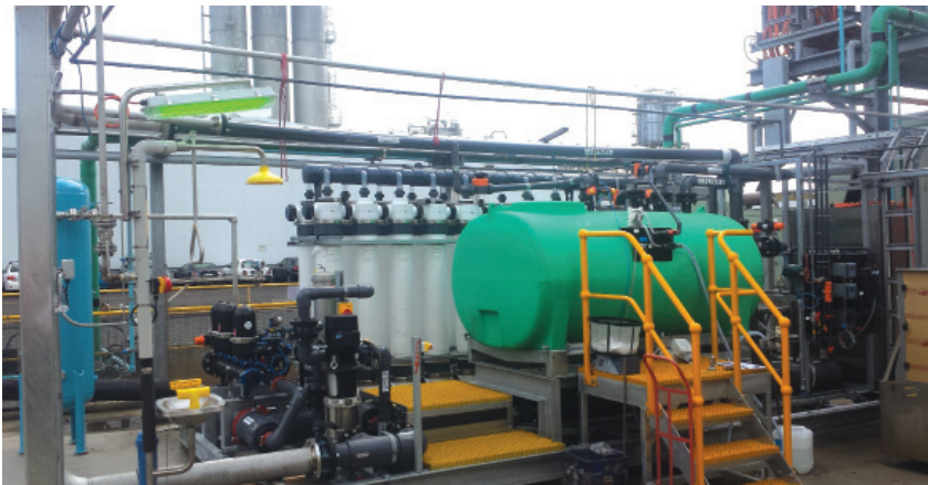
Figure 8. Botany UF skid installed at GTP site.
