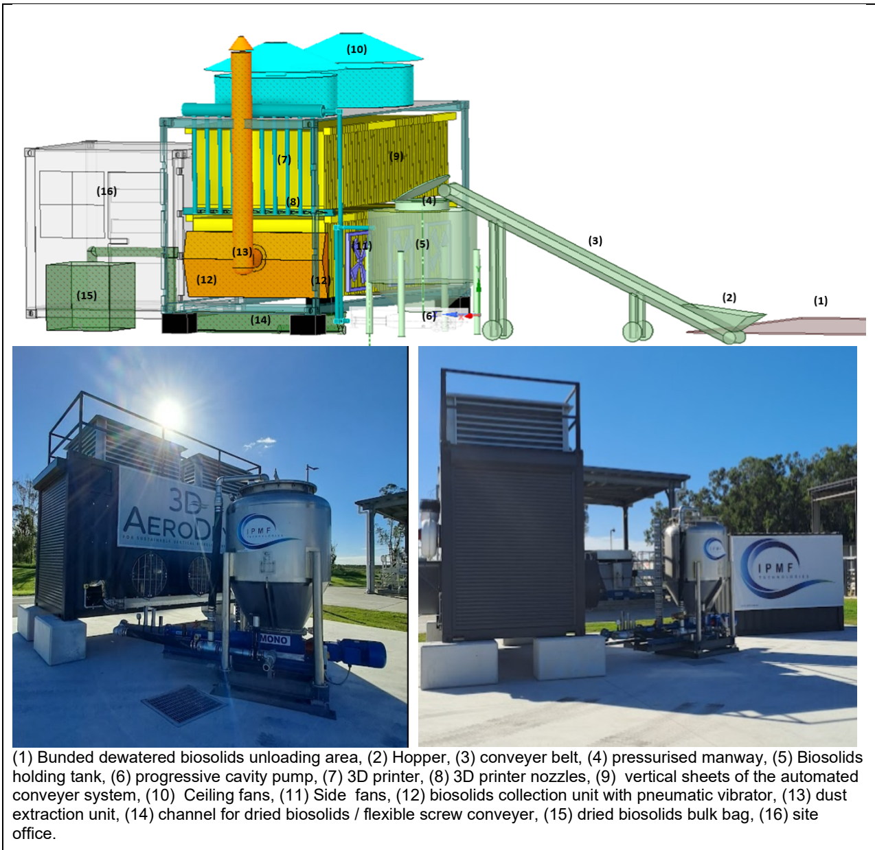
Figure 1: (top) General layout and (bottom) pictures of 3D-AeroDry ® DEMO plant.
