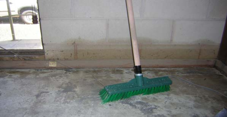
Control room FLOOD line visible (the carpet had been removed)
