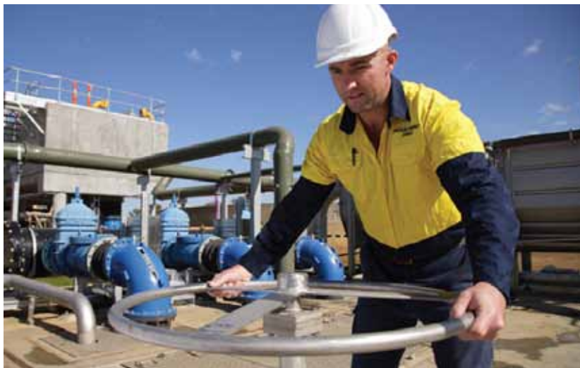
Main Inlet Works
