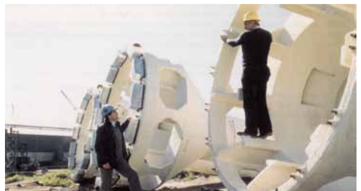
Image 10 - Protective Steel Caissons - Some with Sacrificial Anodes Attached
