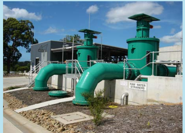
Bray Park raw water strainers
