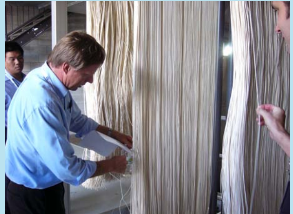
Marty Hancock from Tweed Shire Council points out the membranes at the Bray Park WTP during the technical tour
